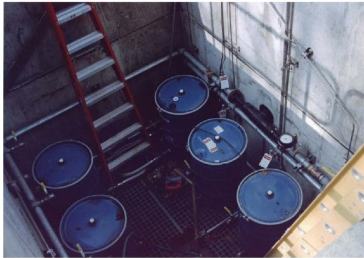
Figure 6: Drums of zeolite positioned in the underground vault. Flexible lines will connect the drums to the header pipe on the right and discharge pipe on the left.
