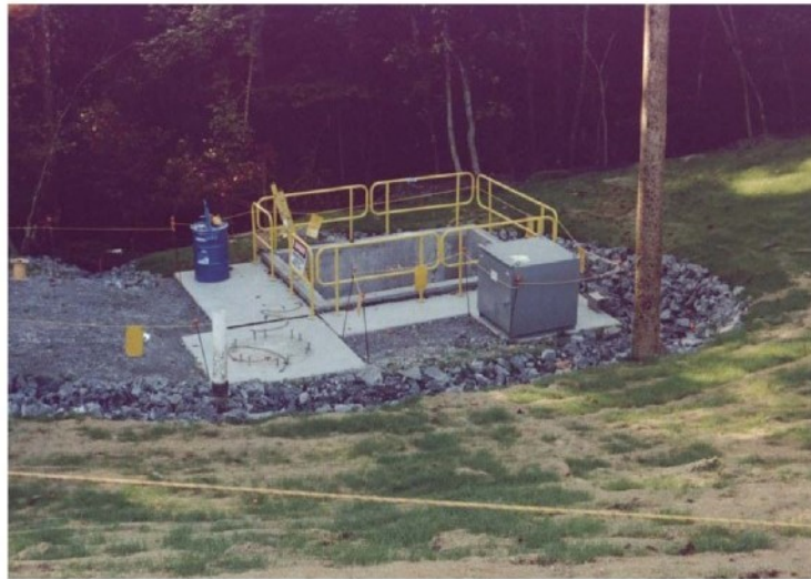
Figure5: French drain to collect the groundwater is under the grass in the foreground. Drums of zeolite are located in the concrete vault. Treated water discharges to the creek in the background.
