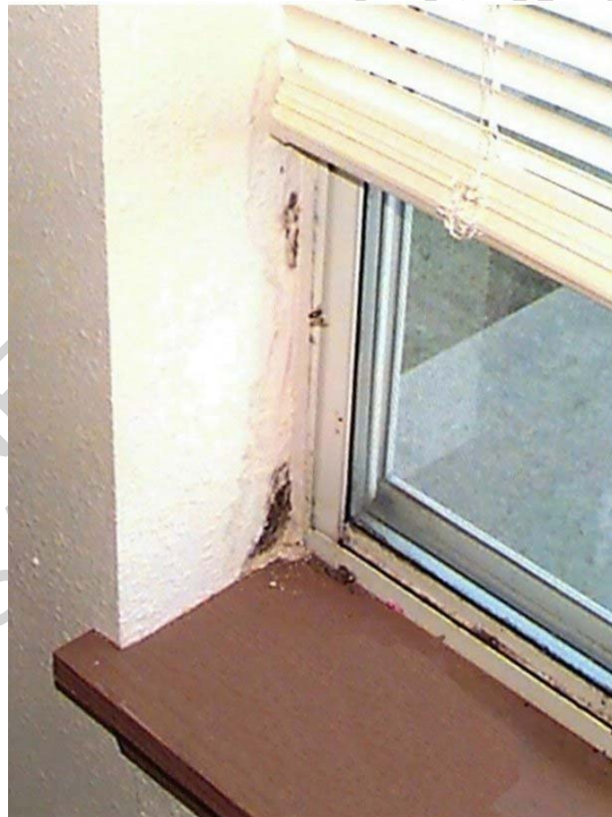
Figure 2: Mold growth at a window jamb, caused by water leakage from the exterior. Photograph courtesy of Mark Meiling, Foresight Home Performance, Wauwatosa, Wisconsin.
