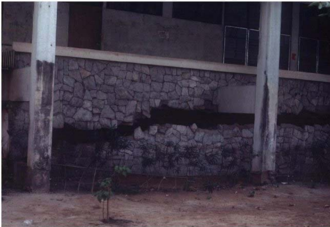
Photo 2: Structural damage due to subsidence of a waterlogged soil (Source: Laker).
