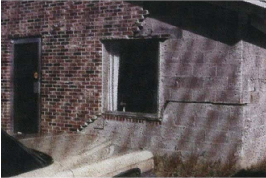
Photo 1: Cracking of a house on swelling clay soil (Source: Muckel, 2004).
